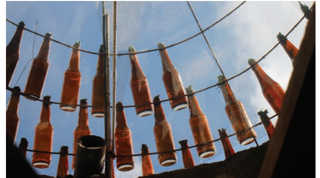
Below: Liter bottles of beer are affixed to a chicken wire and rebar cage to form the cupolas of the domes.
