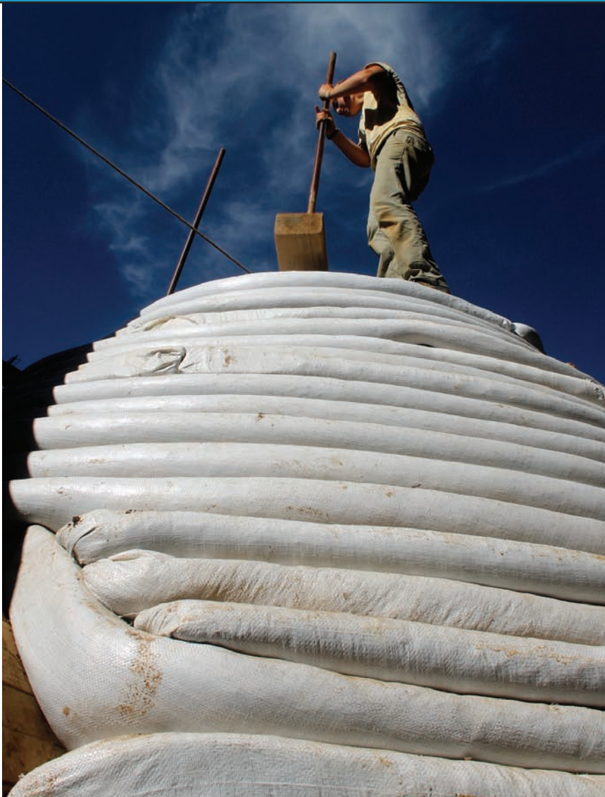
Previous Page: Staff member Bryan Many lays a strip of barbed wire between two courses of earthbags.
